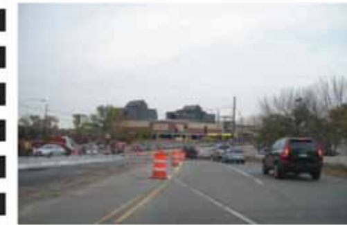
Park Place Blvd, satisfactory for pedestrians, potentially unsafe for cyclists. New multi-use trail under construction south of I-394.
