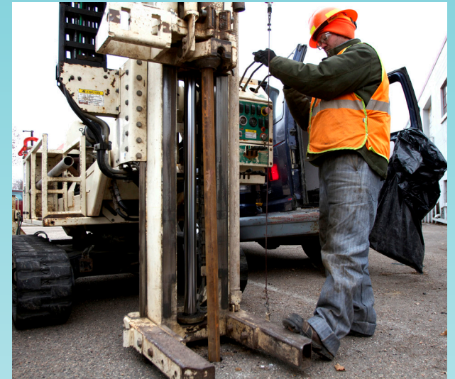
Above, test boring underway related to the Highway 100 and County Road 3 Groundwater Plume.
