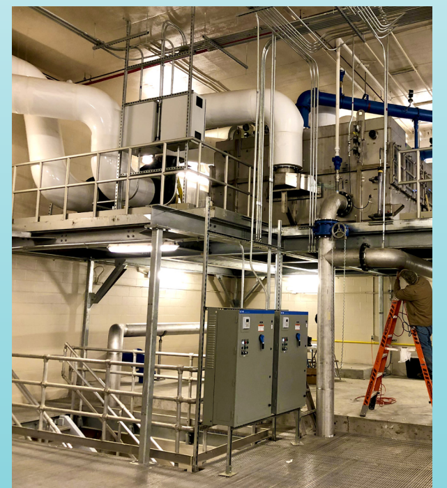
Above, the inside of Water Treatment Plant #4, upgraded to treat VOCs.
