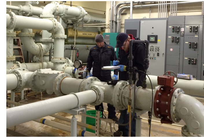
Drinking water treatment plant.
